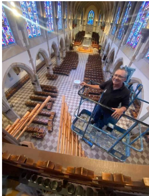
Derek removing pipes from the Nave division at University of the South’s Chapel in Sewanee, TN.
